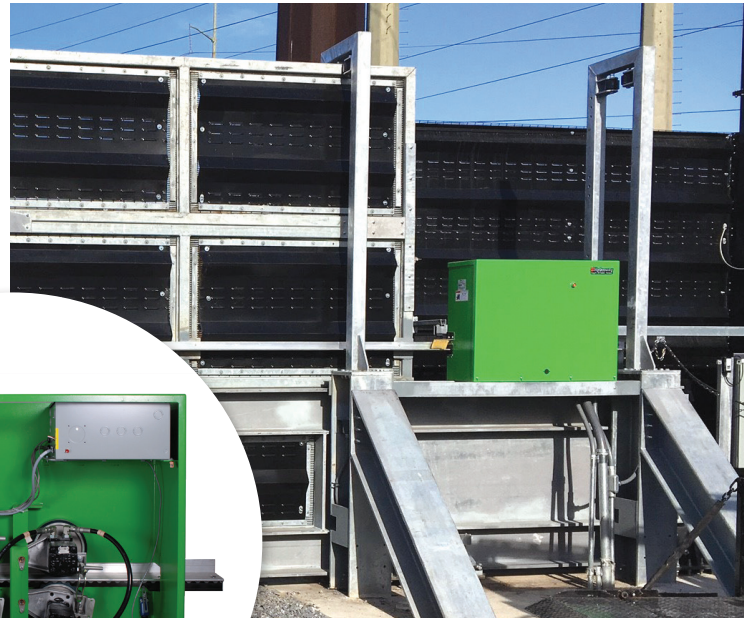
SlideDriver 200 operates crash gate at power substation
